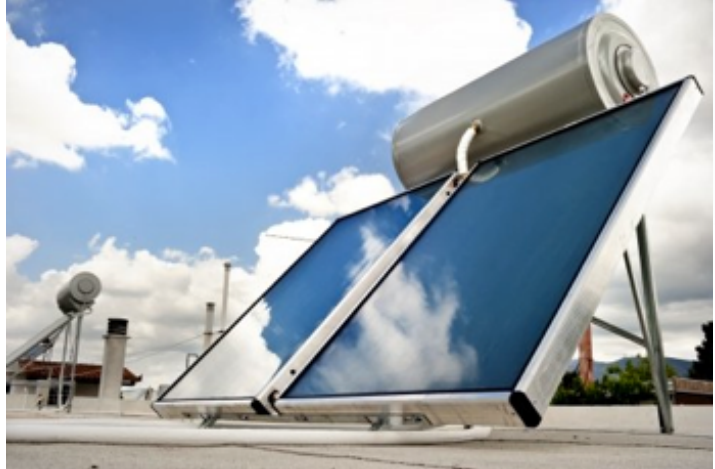
Solar water heater
